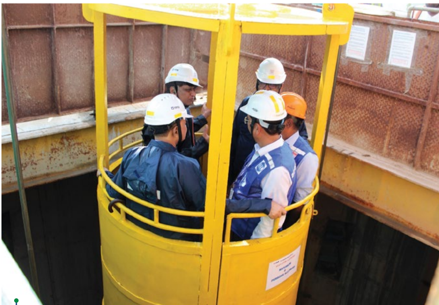
C&MD, HPCL in a review visit to HPCL LPG Cavern project at Mangalore, a testament to our commitment to safety and energy security
